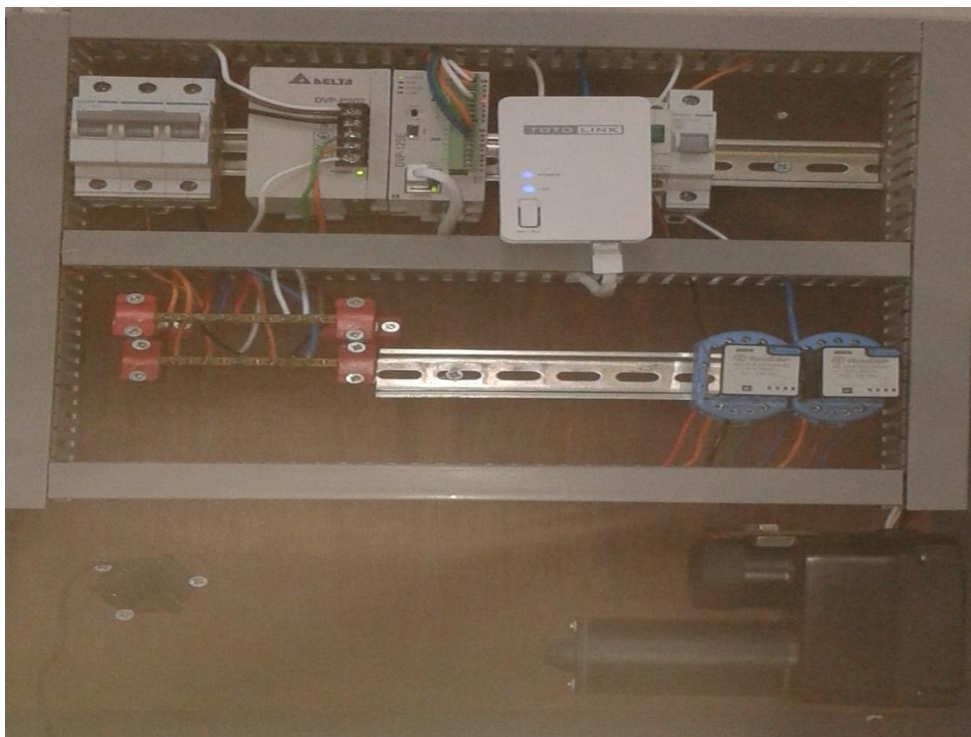
Figure (5.4): Control board of programmable logic control lab.
