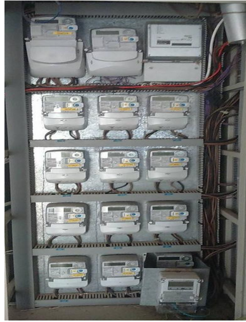
Figure (4.3):The serial connection of Smart meters
